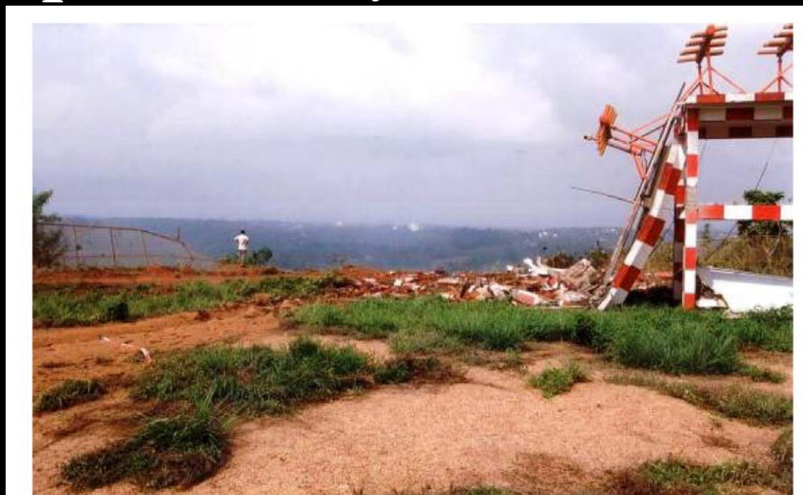
Photo 9: Broken ILS Mounting Structure Due to Impact of Wing
